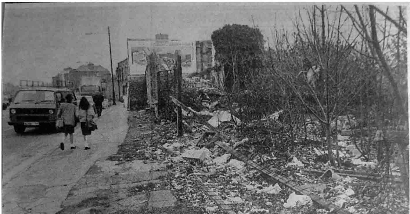
GOING . . . one of the derelict sites demolished to make way for the Clanbrassil Street roadway.
